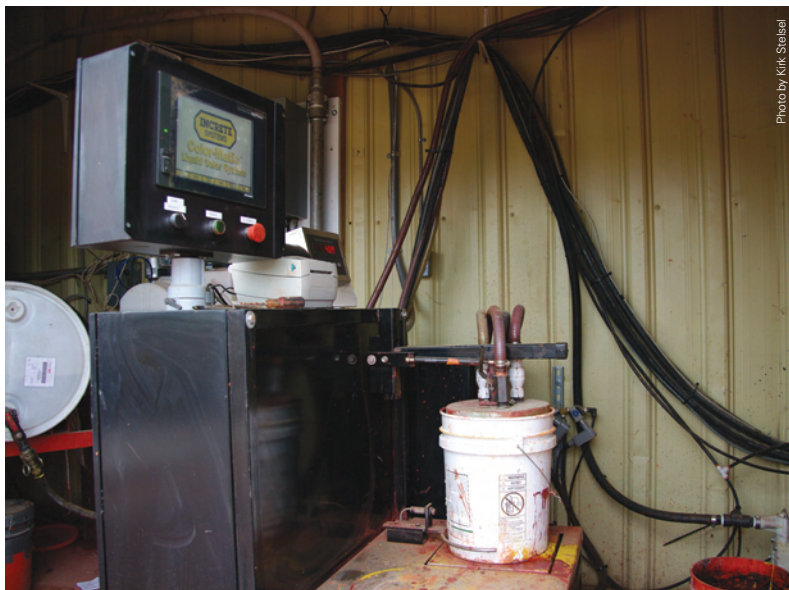
UNIVERSAL PRECAST'S COMPUTER-MONITORED COLORING SYSTEM, DESIGNED BY INCRETE, CAN MATCH ANY COLOR ON THE MARKET.
