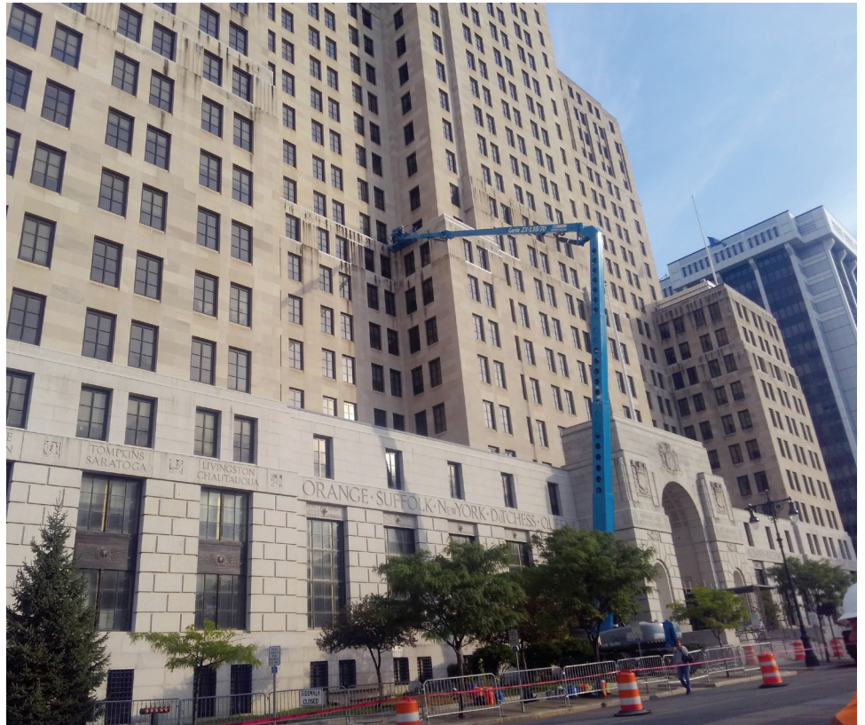
Union bricklayer Dennis Sisson works on the Alfred E. Smith State Office Building in Albany, NY. DeBrino Caulking Associates, Inc. patched stone, did stone Dutchmen repairs, as well as caulking and corrective work on thru-wall flashing on the building.
