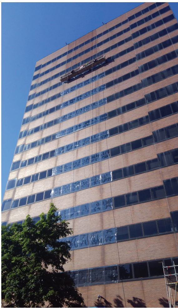
Union bricklayers Walter Doty and Arthur Reed, with DeBrino Caulking Associates, Inc., cut out and recaulked all windows and control joints, reglazed windows and cleaned and sealed the Ten Eyke State Office Building in Albany, NY.
