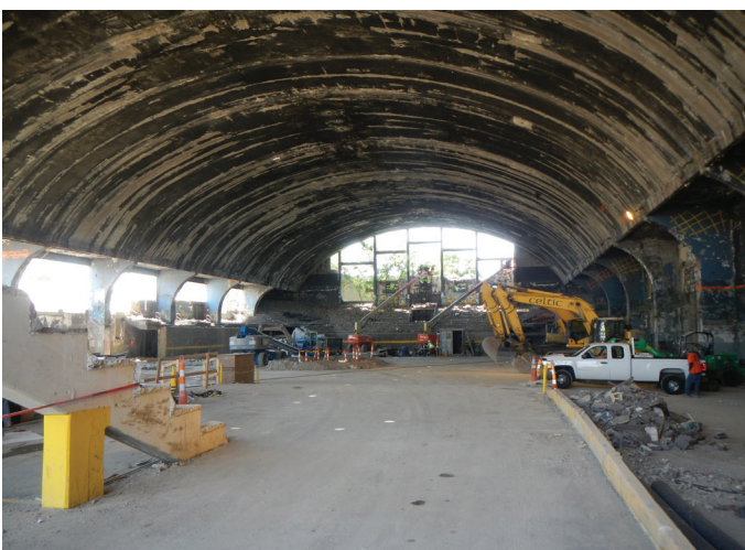
Fig. 2—Thin sprayed concrete panels form the barrel shell roof, which extends 157 ft (48 m) along the length of the arena.
