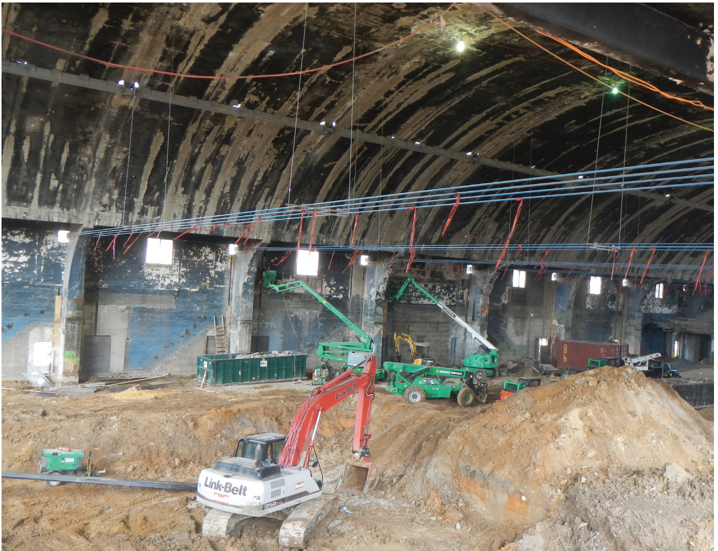
Fig. 4—PT cables installed at column beam locations and supported by temporary hangers.
