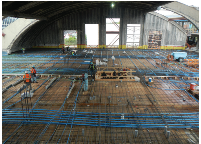
Fig. 7—Cables incorporated into the new two-way PT concrete slab acting as additional reinforcement only.
