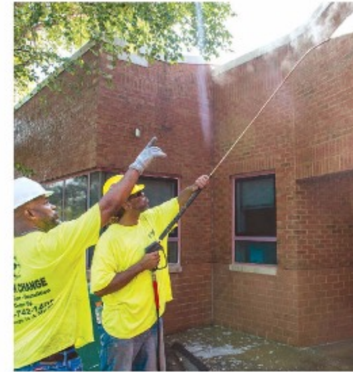
A Sudden Change crew member cleans a brick wall at a newly completed masonry project.
