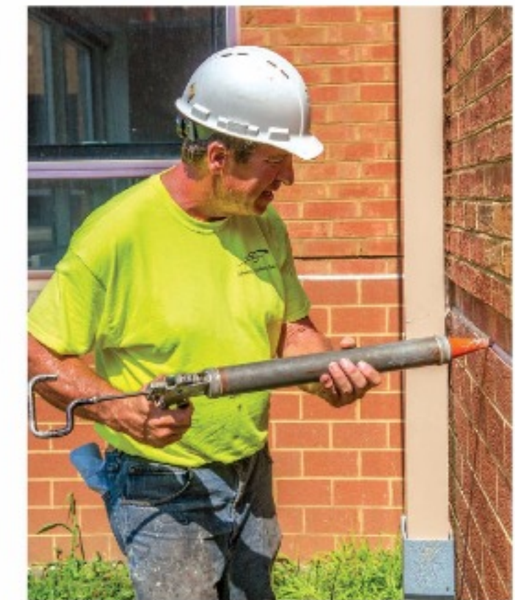
A Sudden Change crew member provides repair work on a masonry project.
