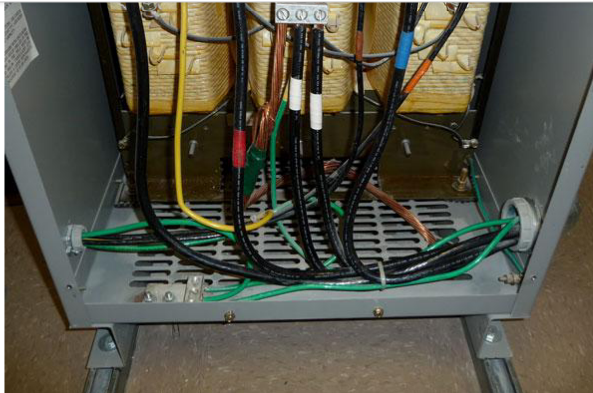
Photo 3. This separately derived system/transformer has a compliant system bonding jumper; however, the required grounding electrode conductor is absent.
