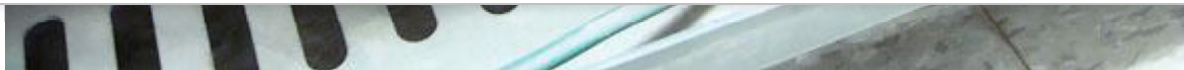
Photo 1. This 8 AWG bare copper system bonding jumper is undersized for this installation. NEC Table 250.66 requires a 4 AWG or larger copper system bonding jumper for 3/0 AWG copper derived ungrounded circuit conductors.
