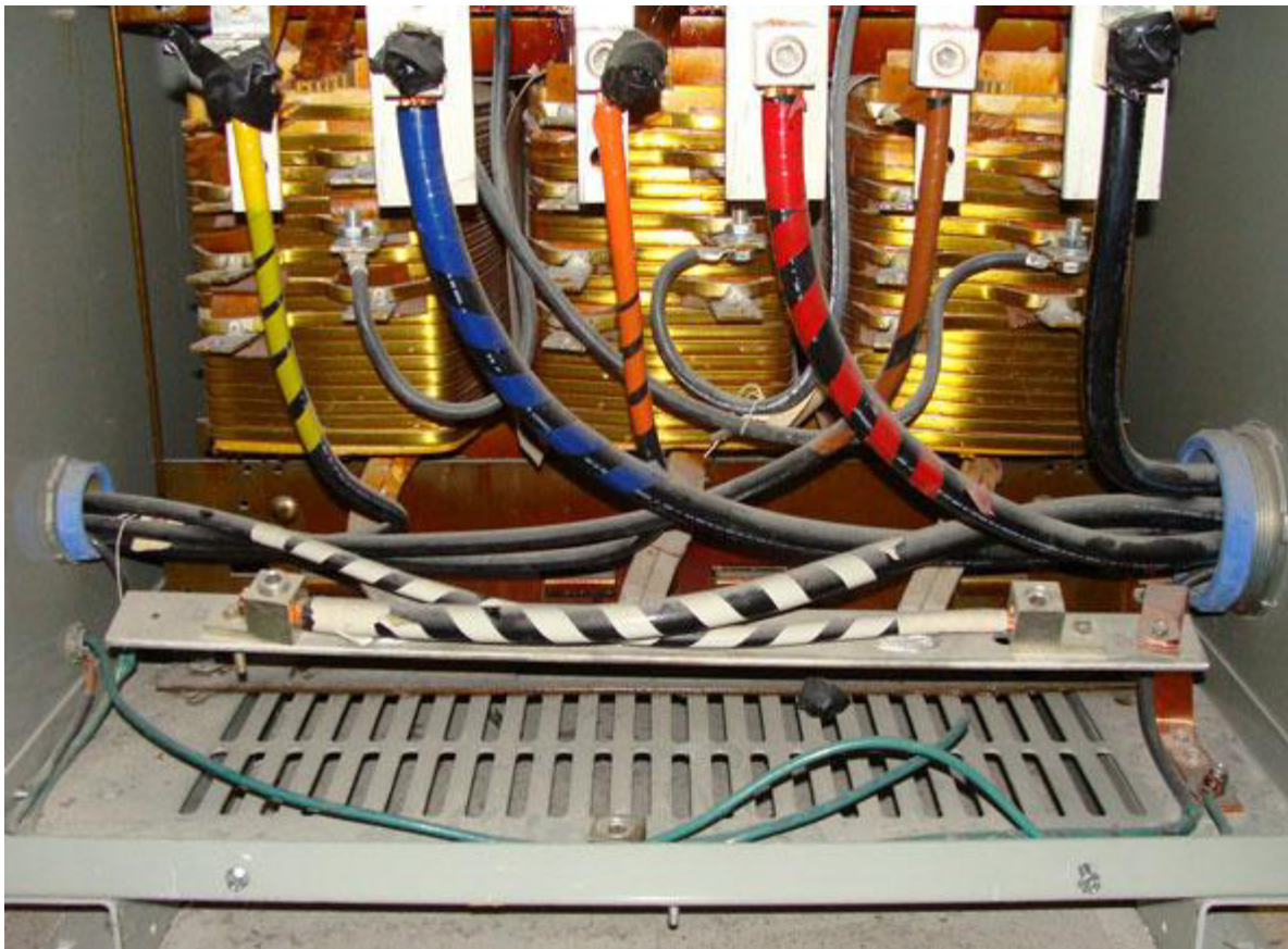
Photo. 2. Note in the photo how the 3/0 AWG bare copper grounding electrode conductor originates from the neutral point XO and pierces through the mesh in the bottom of the transformer enclosure. Because the
