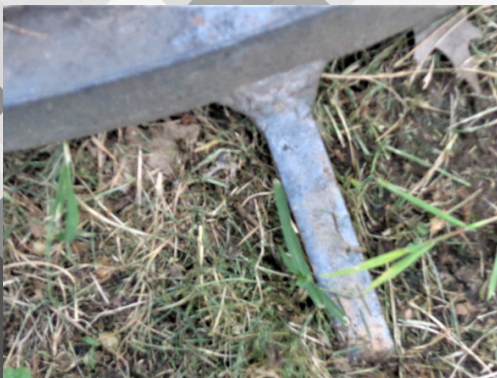
No corrosion or rust on the foundation top plate exposed to the elements since 1994 at Marietta College.
