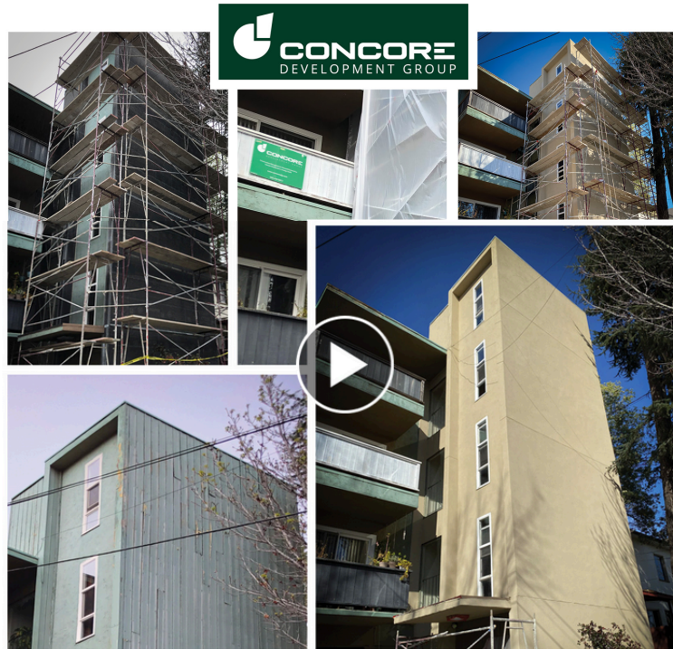
DWIGHT WAY EXTERIOR — BERKELEY • CA Stucco Upgrade to 4-Story Residential Apartment Building
