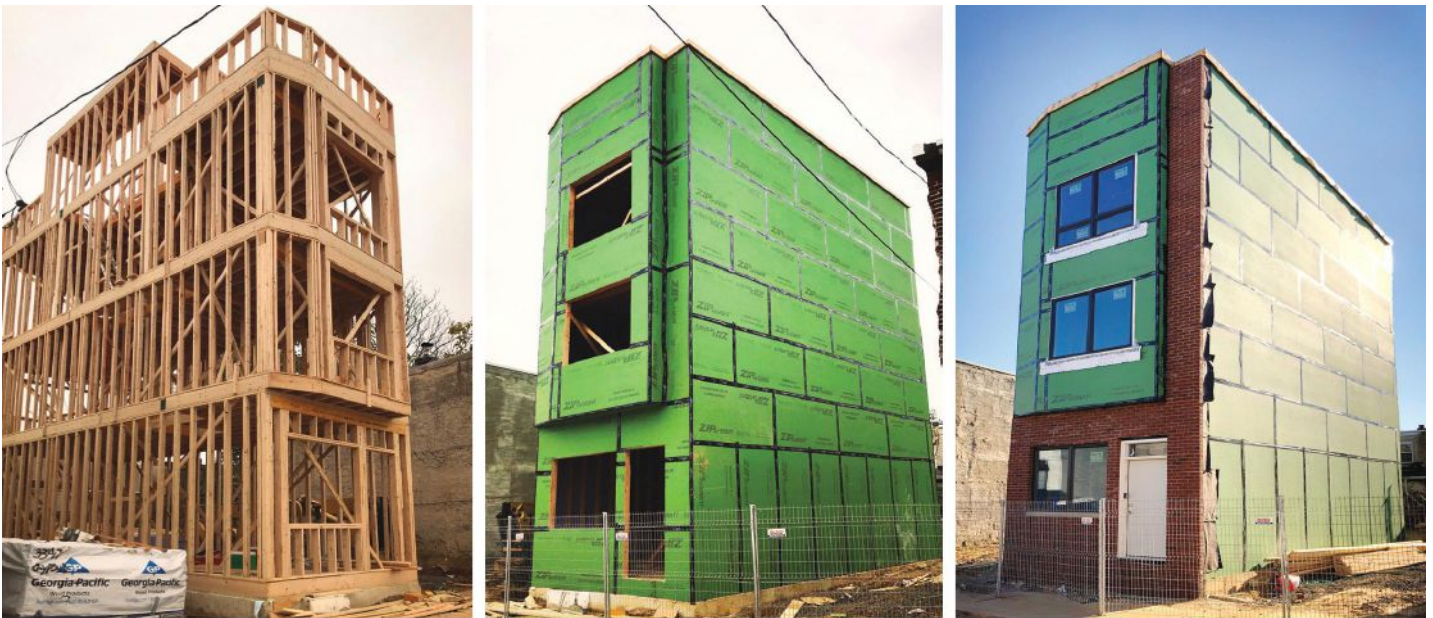
The Designblendz Construction team completes framing and installs waterproof Zip System® sheathing, windows and brick for a South Philadelphia row home project.
