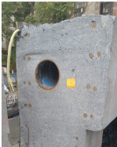
Encapsulation around reinforcement, embedments and encasement of a waterbarrier (on right lower side)
