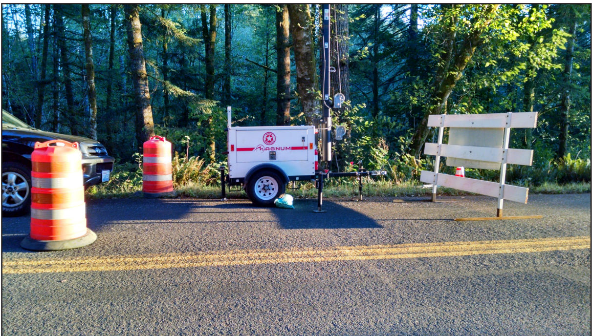
Traffic control and closure barricades were part of the emergency replacement project.
