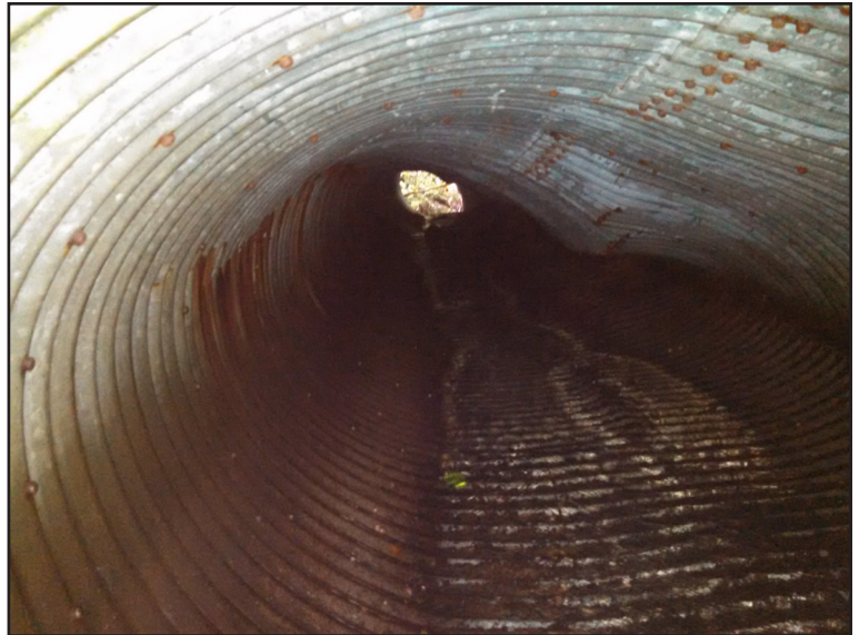
Another look inside the failing culvert.
