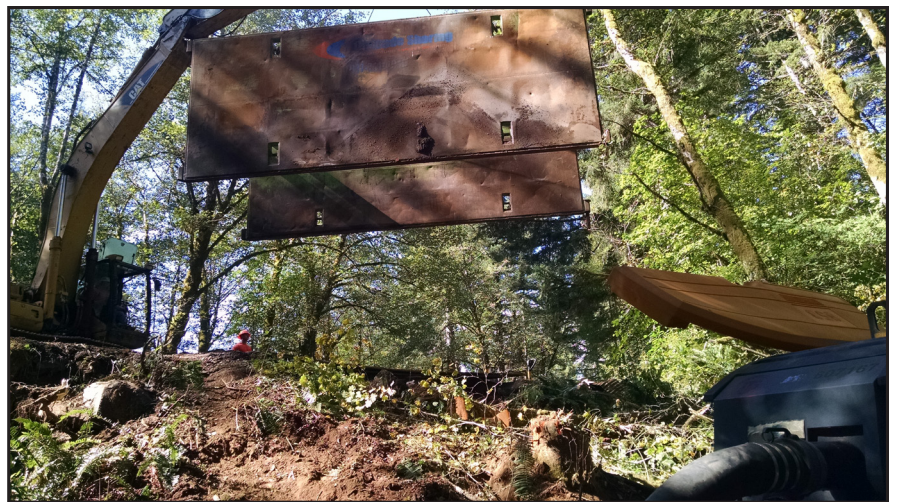
Metal plates were used to shore up a trench for the replacement culvert.
