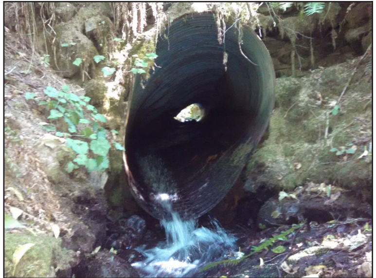
The collapsing culvert under Falls Road, one month before it was replaced in early October 2014.
