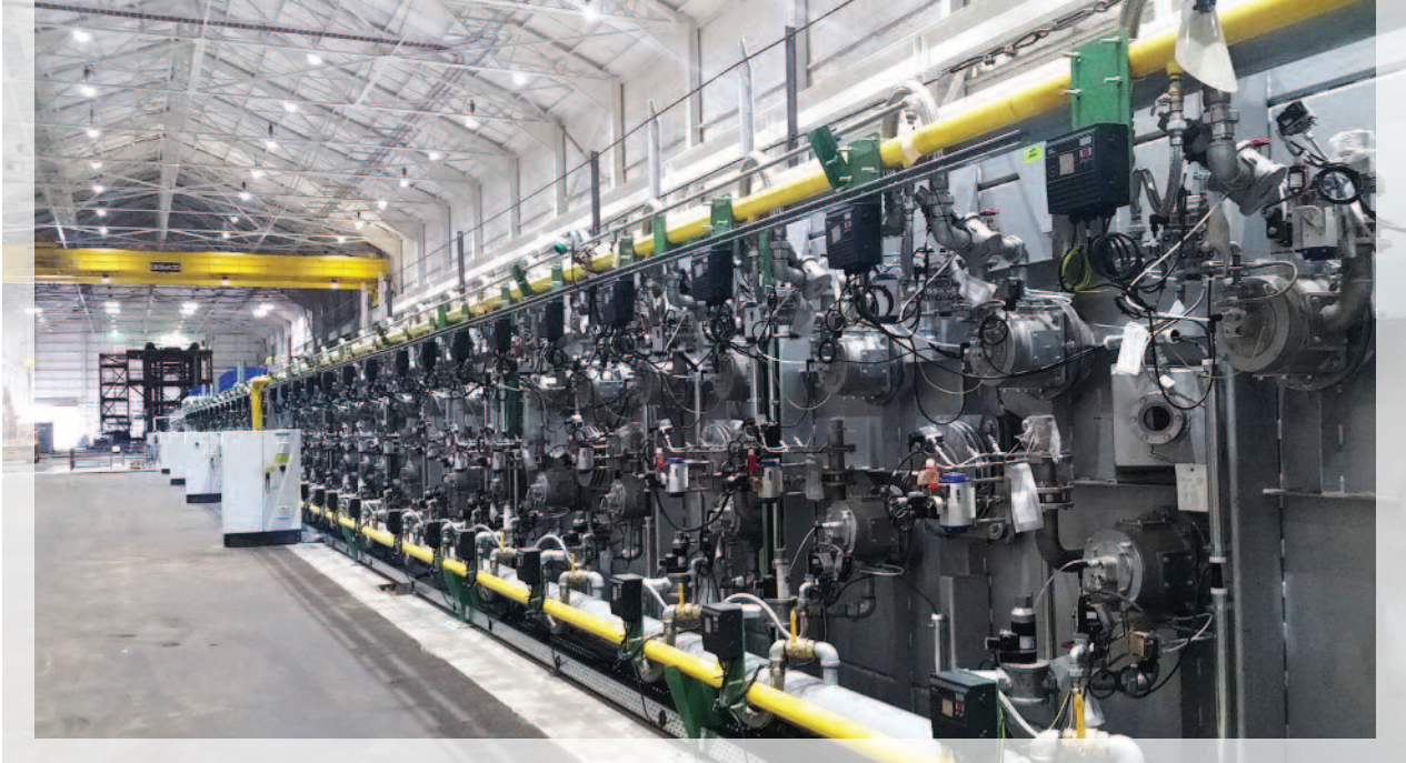
Electricians and pipefitters finished installation of 124 radiant tubes in the furnace heating sections for HyCAL.
