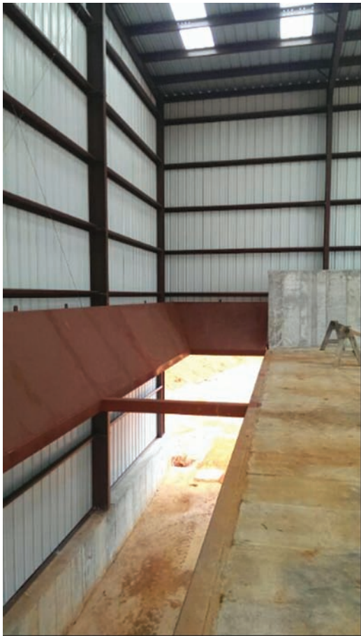
Push pit at the City of Bainbridge, GA Transfer Station. Photo courtesy of sowegalive.com
