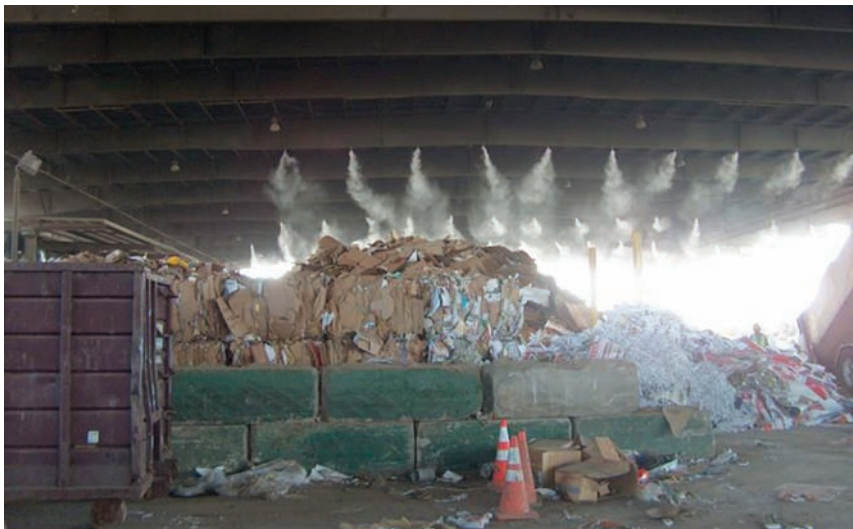
Figure: Misting system at a transfer station. Photo courtesy of NCM Odor Control.
