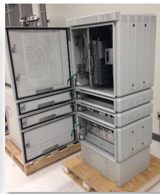
Equipment & Battery Cabinet
