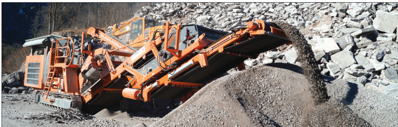
A Rockster impact crusher R1100D recycles 100,000 tons of highway concrete, which is reused for stabilization and fillings in road construction.
