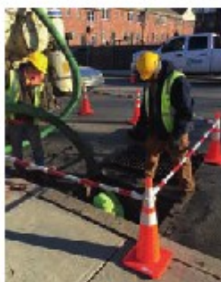
The contractor ISS builds, cleans, and inspects catch basins for the Stormwater Authority of Chester. Mason Negvesky (left) of ISS helps clean and inspect an existing catch basin. Photo by Corvias
