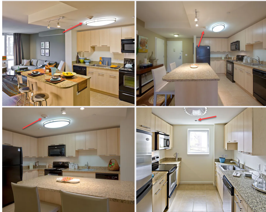
Figure 9 - Heat Detector Mounted Location
