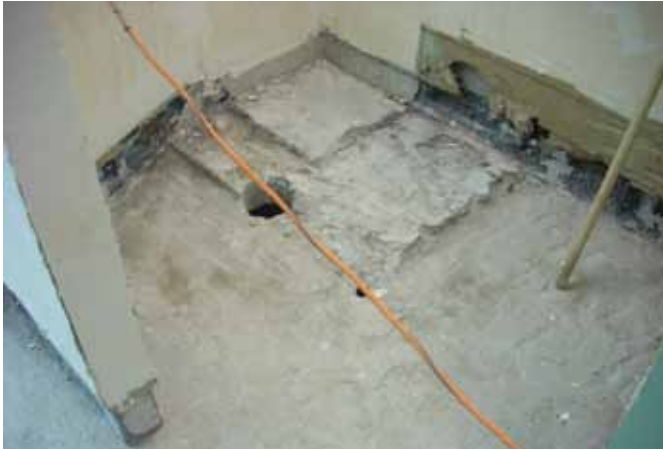
ABOVE ▲ “When we demoed the existing tile deck we discovered a 5" (12.7cm) sand mortar aggregate. This was unusable for our specified coating application and the floor had to be resloped.”
