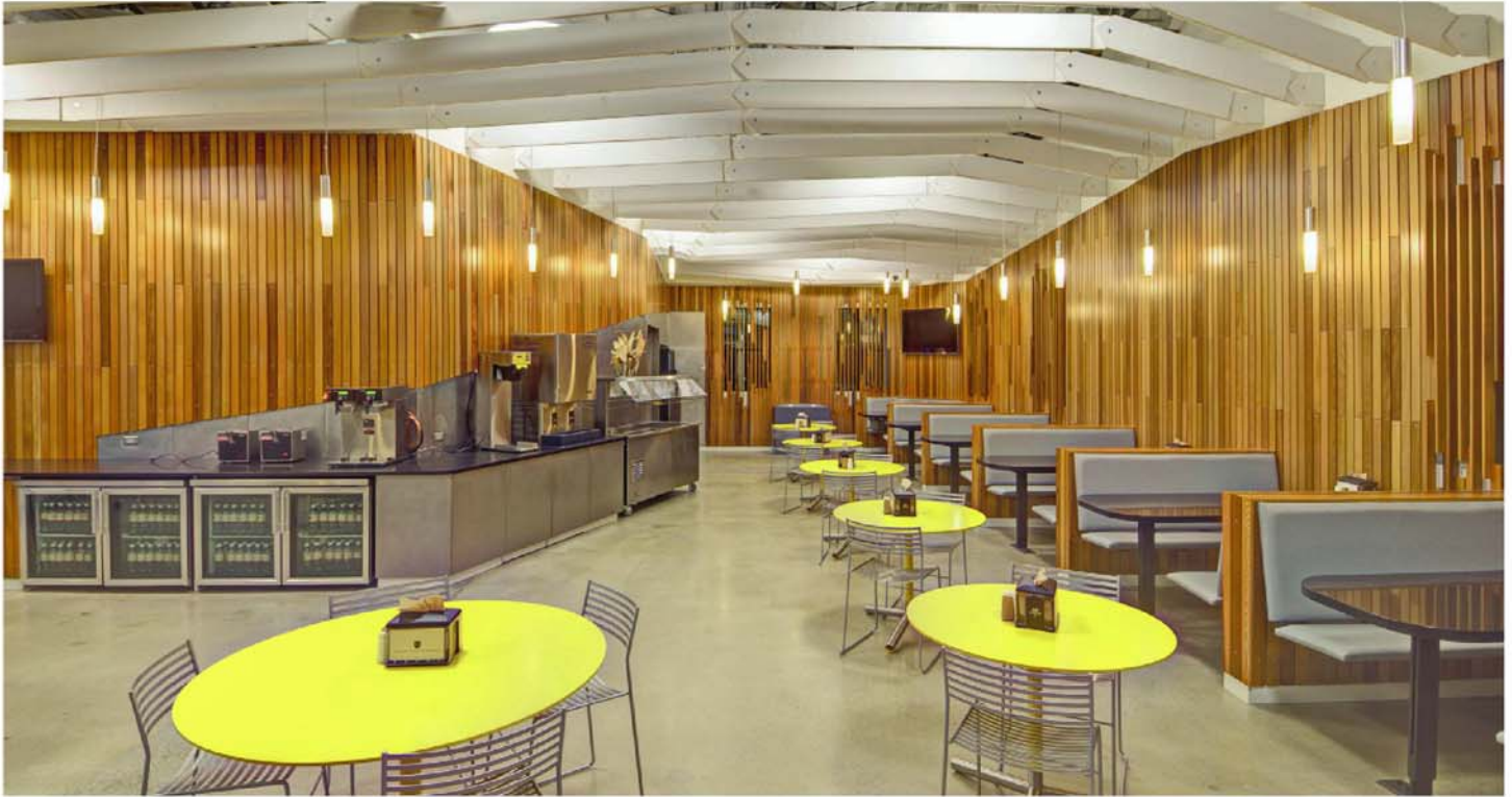
Our scope of work in the Café area included the banquette seating with granite tops and bases, stainless steel wall paneling, stainless steel cladding on the base cabinets along with the cedar paneling and ceiling baffles.
