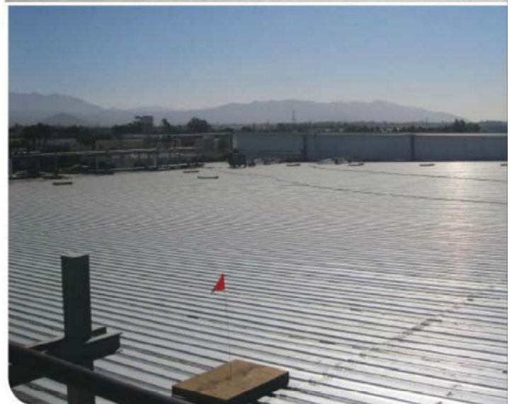
The 4-7-person Cool-Roof Systems crew had much to do to help turn a building into a cold storage facility for avocados. They used spray polyurethane foam (SPF) and coatings to get the job done.
