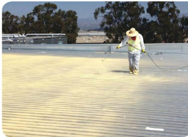
Typical jobs require 1–1.5 inches (2.5–3.8 cm) of foam, but this job required 5 inches (13 cm), according to co-owner Lyle Orth. The crew filled all flutes with ~940,000 board feet (2,218,153 L) of SPF.
