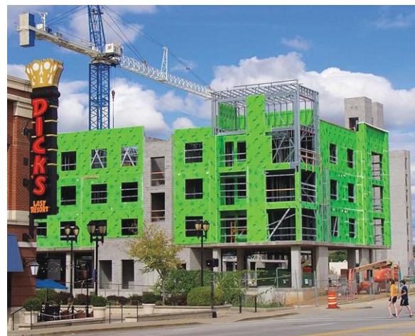
Aqua on the Levee, a waterfront apartment community in Newport, Kentucky, was built with Tri-State’s cold-formed components.
