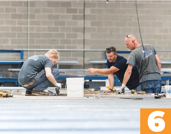
Christian Hodges (from left), Casey Hillerich and Hank Basham assemble a truss in Tri-State Cold-Formed Steel Components' truss shop.
