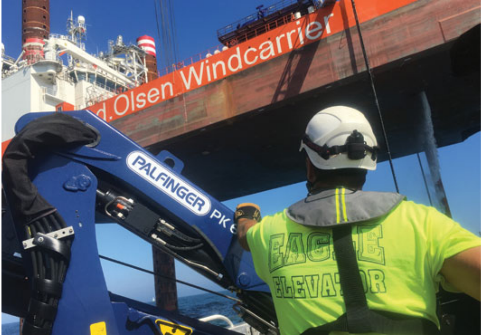
Eagle Elevator's Walt Farren, lead elevator mechanic, installs the elevator systems for the Block Island Wind Farm, the first commercial offshore wind farm in the U.S.
