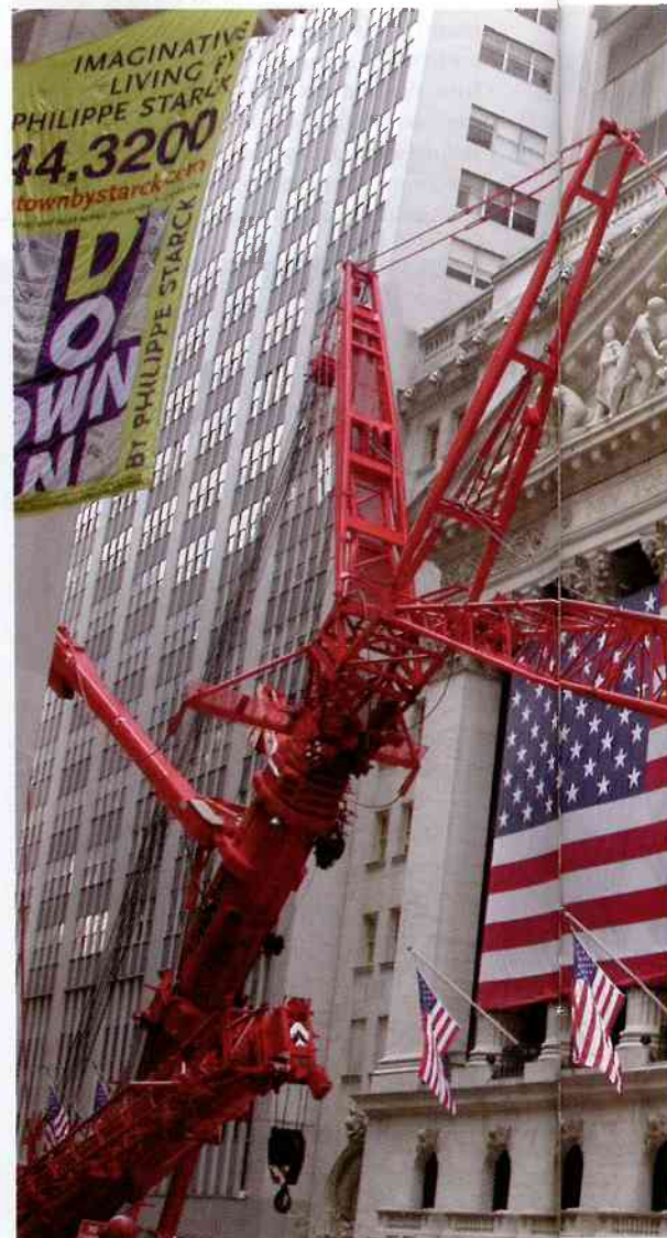
At the New York Stock Exchange, Cranes, Inc. uses a Liebherr LTM 1500 with luffing jib and Y-Guy Superlift to erect new emergency generators
