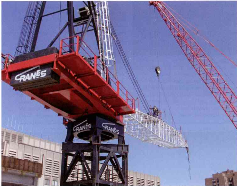
Cranes, Inc. removes its Favco 1000E tower crane from the roof of Bellevue Hospital in Manhattan with a Liebherr LTM 1500
