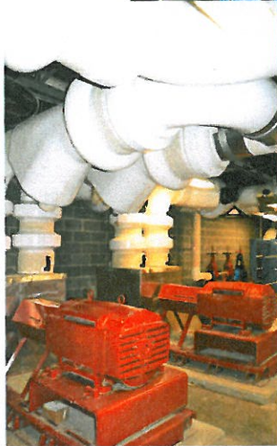
Bell & Gossett pumps.
