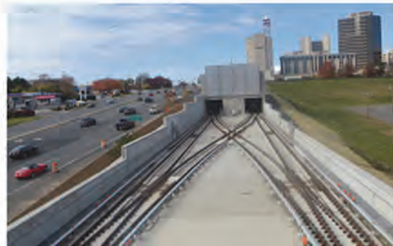
Shapiro & Duncan installed mechanical systems for the Dulles, Va., Metro Silver Line Extension.
