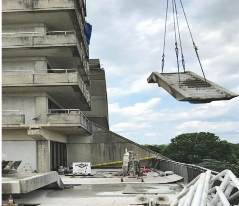
CHESCO Coring & Cutting Inc. uses a saw cutter and crane to remove large concrete pieces from the structure at Cokesbury Village retirement community in Hockessin, Delaware. The project involved cutting and removal of balcony walls around a nine-story building.
