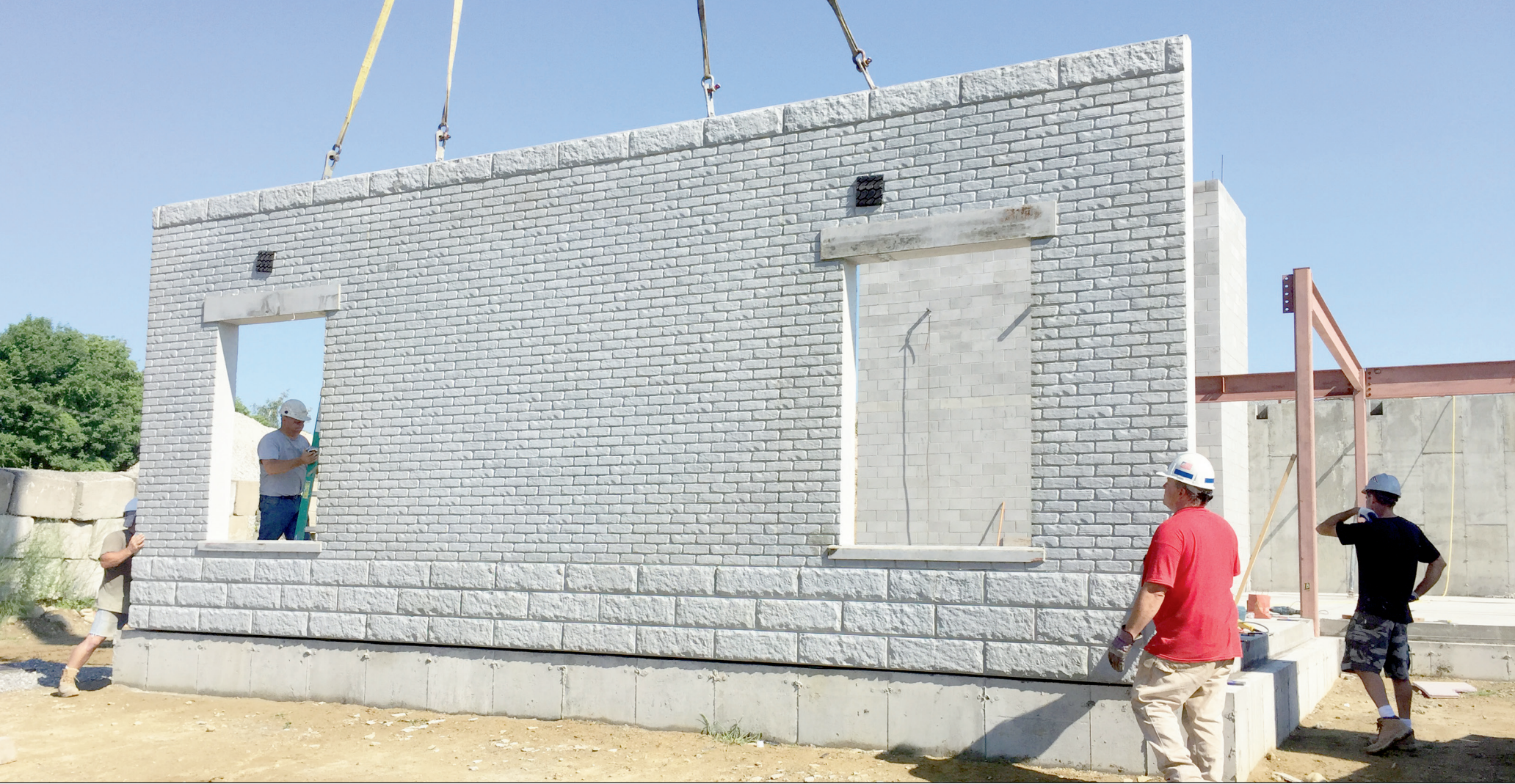
Shea Concrete cast the panels with facades simulating brick work over granite blocks and solid lintels over doors and windows.
