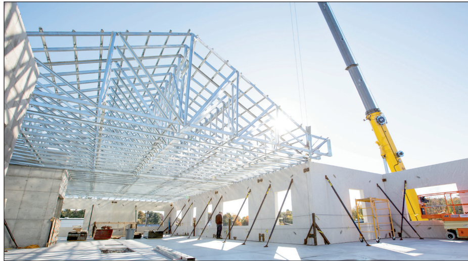
A pre-engineered light gage metal roof truss is ready to support the standing seam metal roof deck. Note the braced precast wall panels. Thirty panels were erected to form the shell of the new building.
