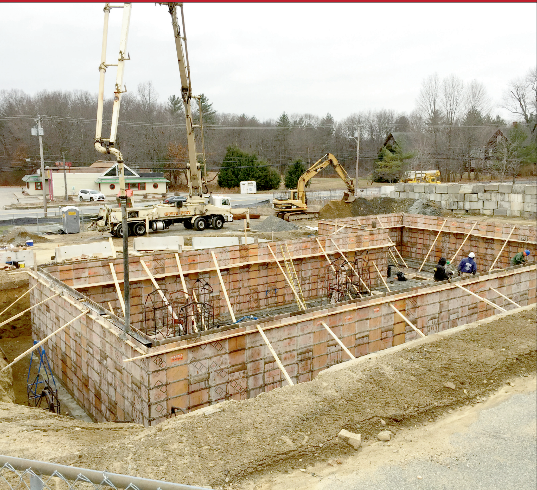
Independent Concrete Pumping conveys ready mix to Bammco crew placing concrete in foundation wall forms for new Shea Concrete headquarters in Amesbury, Massachusetts.
