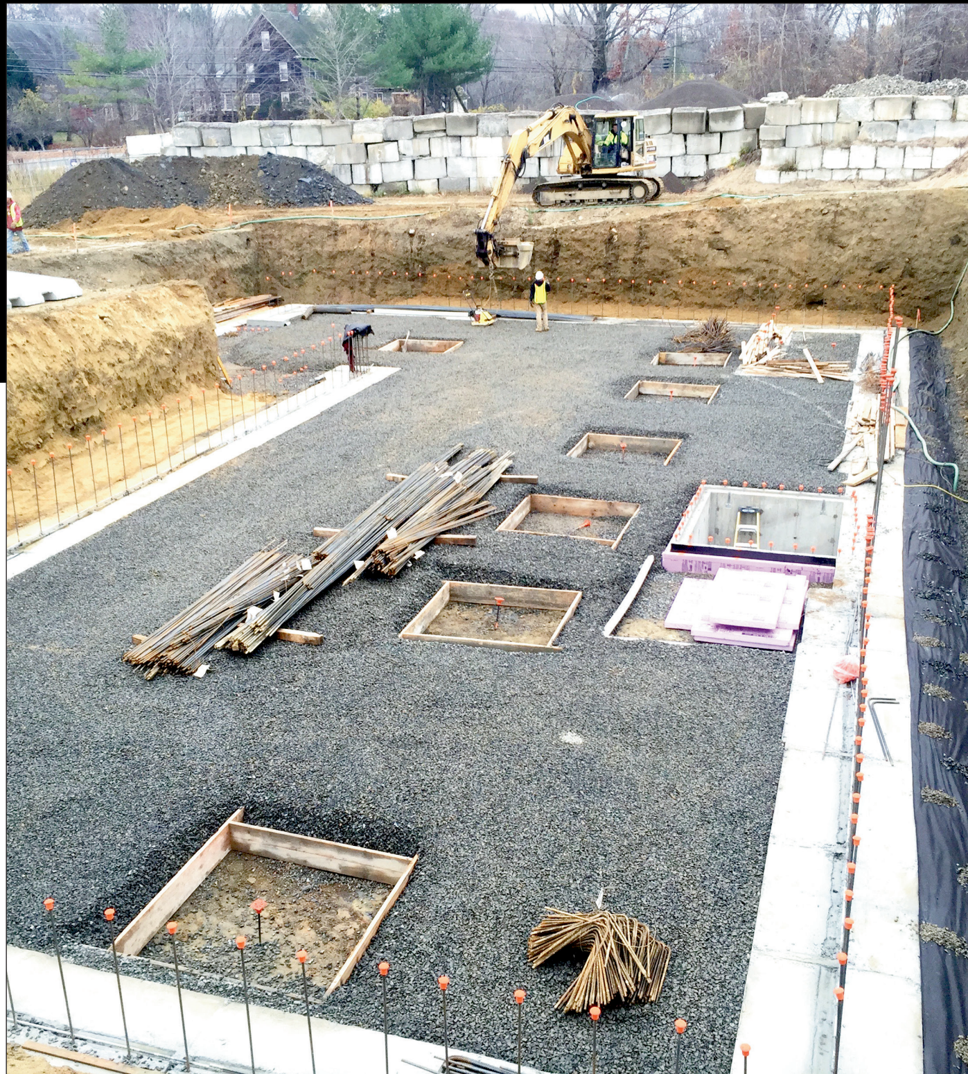
Site photo shows stone bed for building’s basement slab-on-grade, and footing forms for six structurally isolated HSS columns, with Unit Construction’s Caterpillar 315 working in background.
