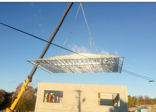
Crane lifts a section of prefabricated roof truss in place on top of wall panels.
