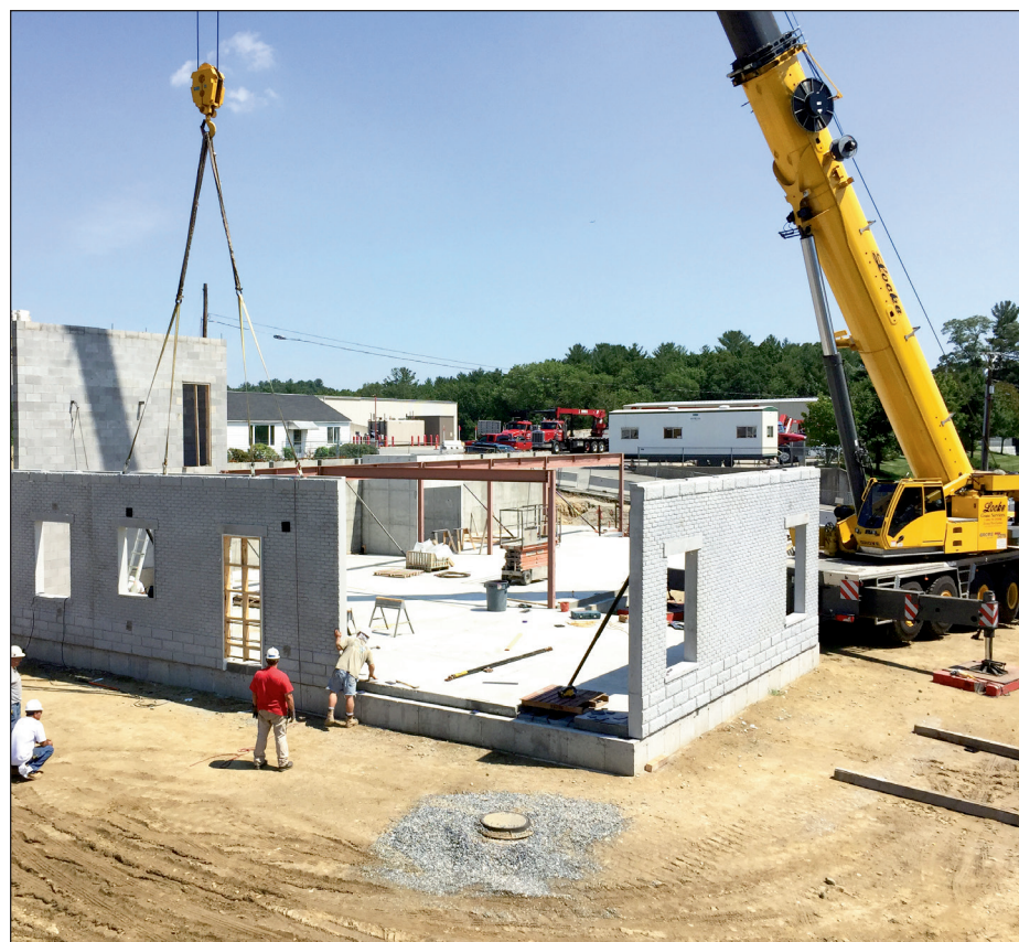
Locke’s 250-ton Grove crane steadies precast panel as Saurman crew guides it onto floor slab’s shiplap recess. Thirty panels were erected to form the shell of the new building.
