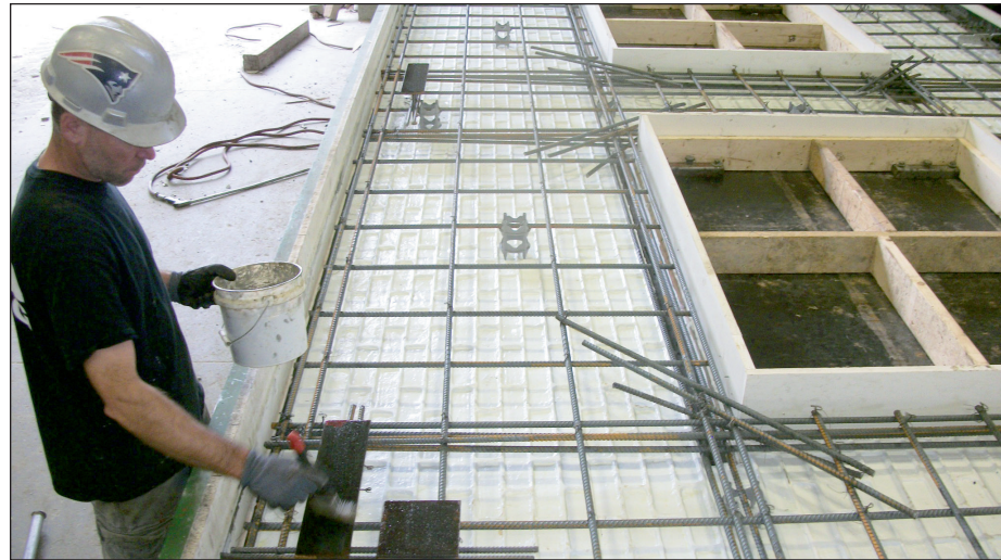
Inside Shea Concrete's NPCA-certified plant, steel connecting plates are placed on wall panel forms before concrete is cast.
