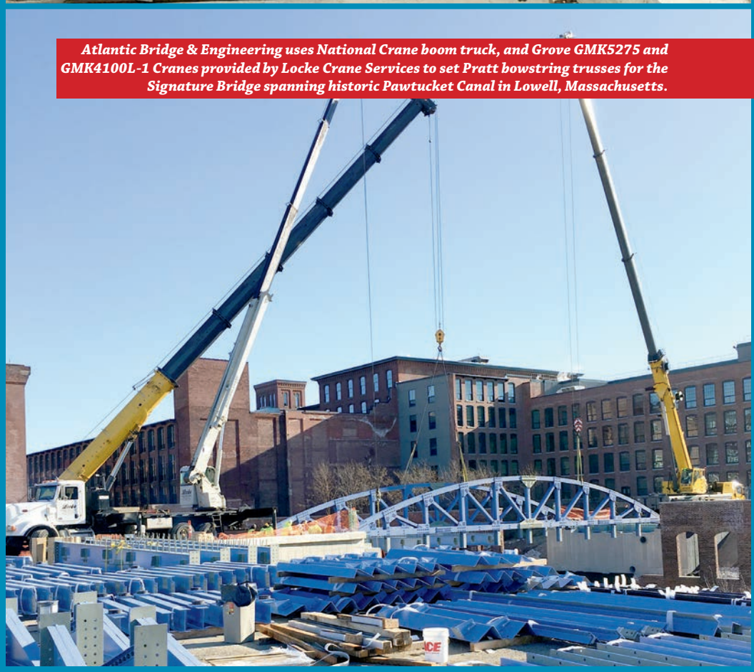
Retaining wall forms for the $7.6 million Signature Bridge are filled with ready-mix concrete.
