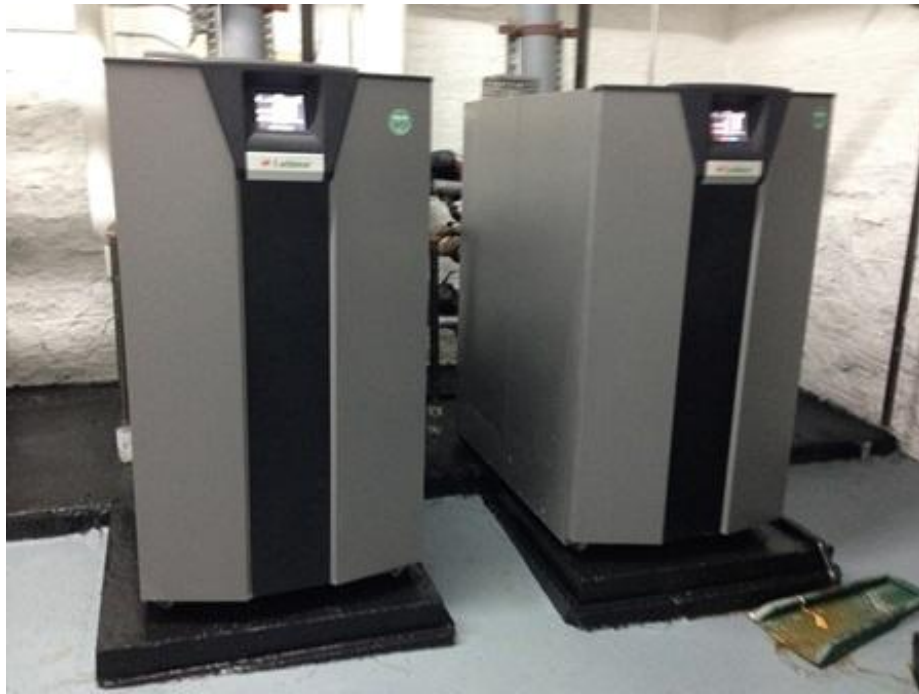
Lochinvar Boiler System
