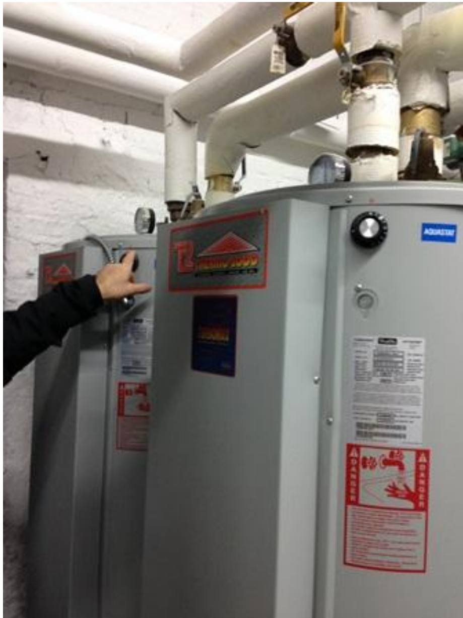
Adjusting water temp settings
