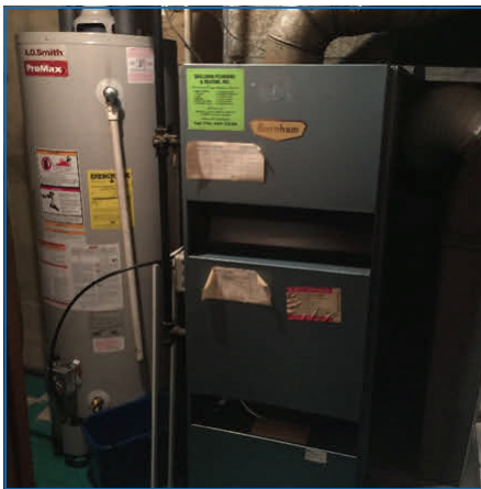
Old domestic hot water maker and furnace
