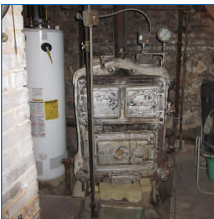
Old boiler covered with asbestos
