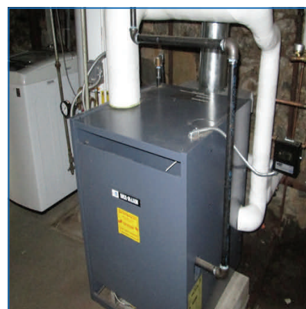
New energy-efficient gas steam boiler
