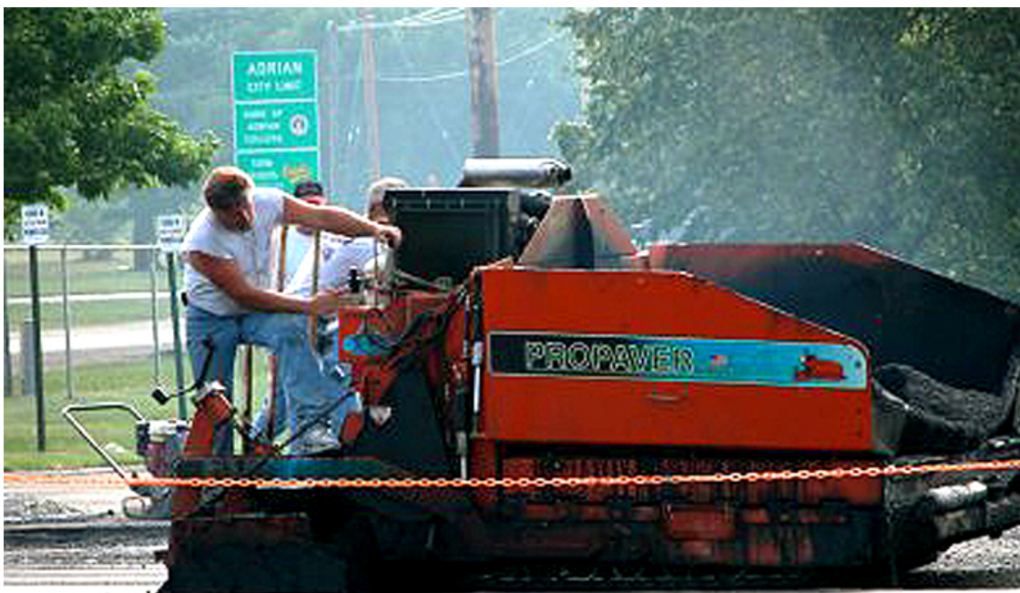
Crew members from Belson Asphalt Paving work on the Merillat Factory in Adrian. The versatile crew can undertake a broad range of projects.
