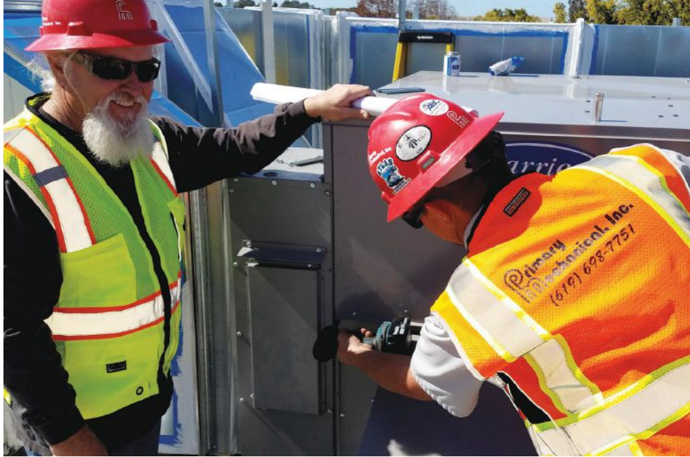
Primary Mechanical, Inc. prepares for the start-up of a Carrier® air conditioner unit.
