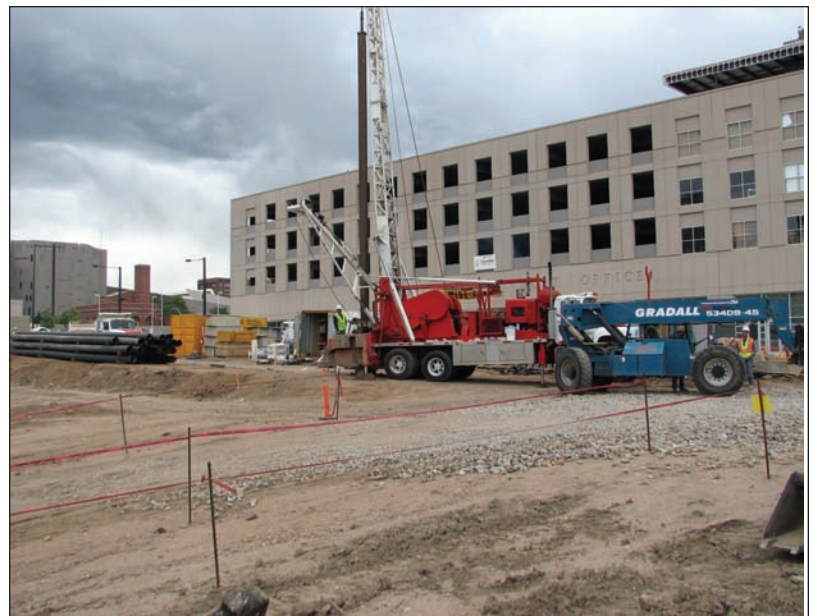
A bucket rig was used at the Denver Justice Center excavation and construction site to drill the boreholes for the well. In all, 30 boreholes were drilled.
