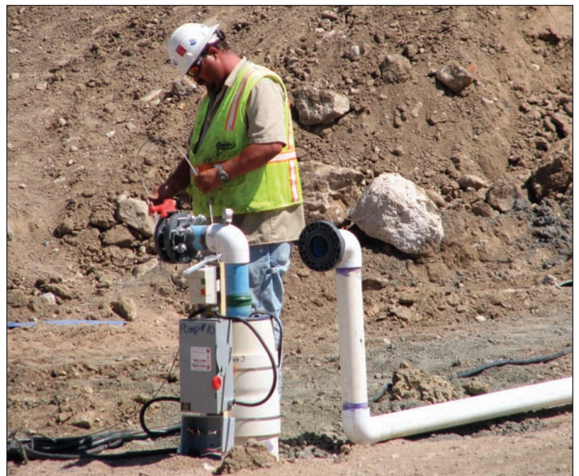
A TerraFirma employee works on wellhead piping at the Denver Justice Center job site. Ten dewatering wells were installed at the job site.
