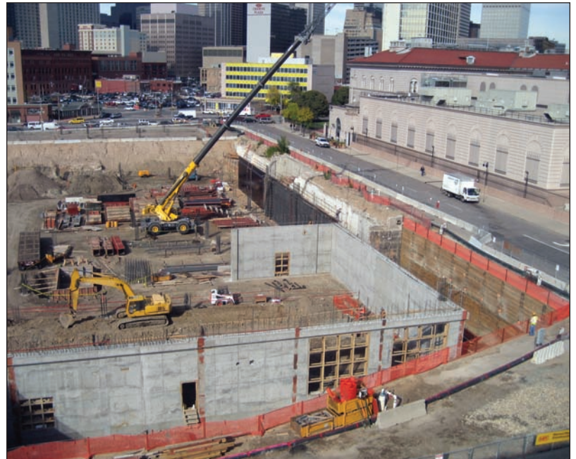
A view of the Denver Justice Center excavation and construction site with the dewatering system visible along the perimeter of the excavation. The project is about the size of a city block and extends approximately 32 feet below ground surface. The water table is located approximately 15 feet below the surface.
