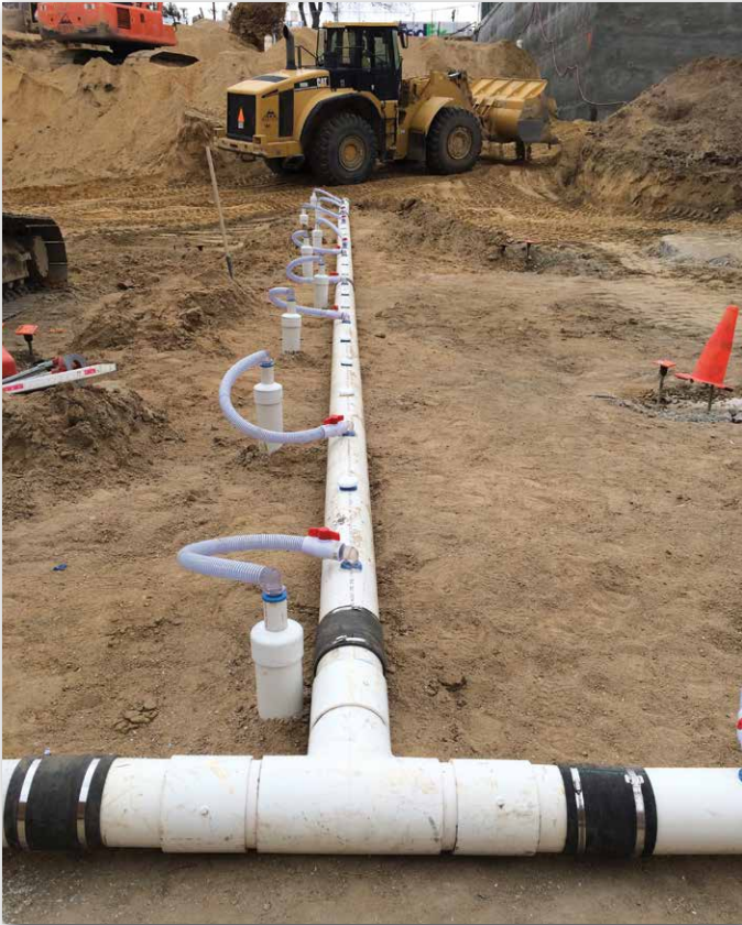
Completed installation of the PVC mini-vacuum well- assembly following drilling of the borehole, utilizing track mounted Geoprobe hollow stem drilling rig.
