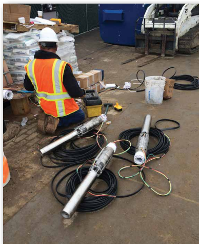
Electrical submersible pumps were placed near the bottom of each dewatering well.
