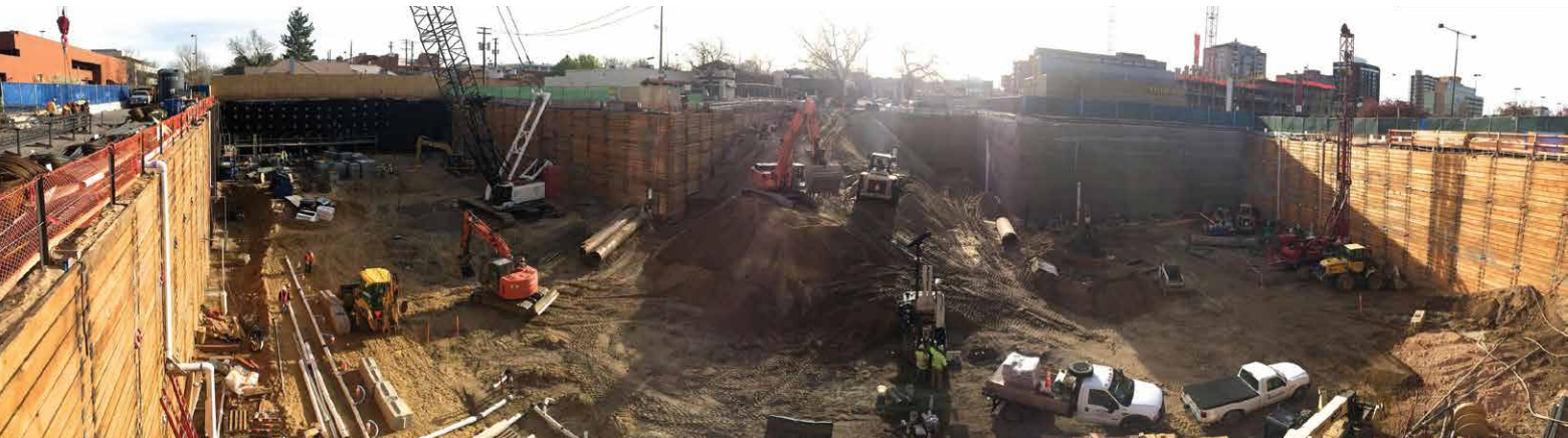
TerraFirma Earth Technologies installed an innovative dewatering and ground water treatment system at 100 Saint Paul, a retail and office development in the rapidly expanding Cherry Creek business district. The firm has made Denver a permanent home to a satellite office.
