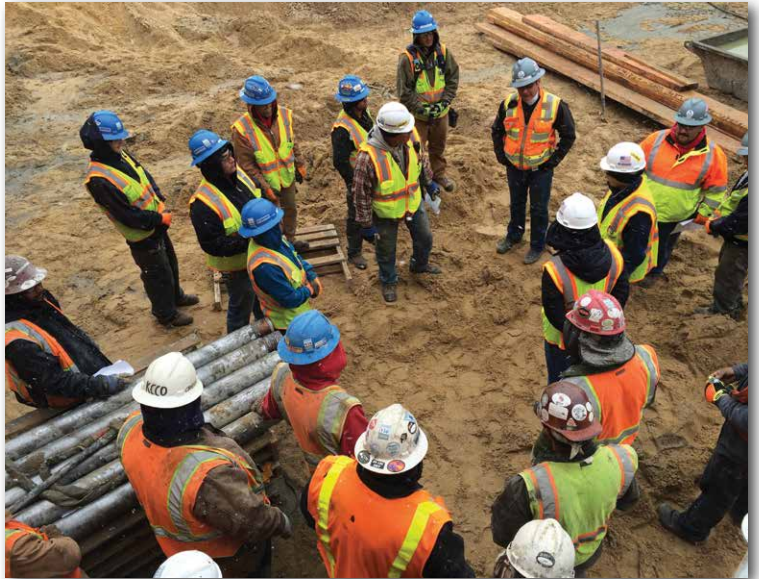
Safety meeting. TerraFirma provides ongoing training and certification for its crew members. All safety initiatives are continuously reviewed and updated to keep employees proficient in new safety policies and procedural methods. The firm calls this plan "Target Zero", and its goal is to achieve zero accidents and injuries during every dewatering project.
