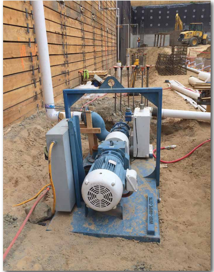
TerraFirma utilizes Holland's Rotary Lobe wellpoint pump for its mini-vacuum well dewatering system. The traditional deepwell dewatering wells can be seen in the background.
