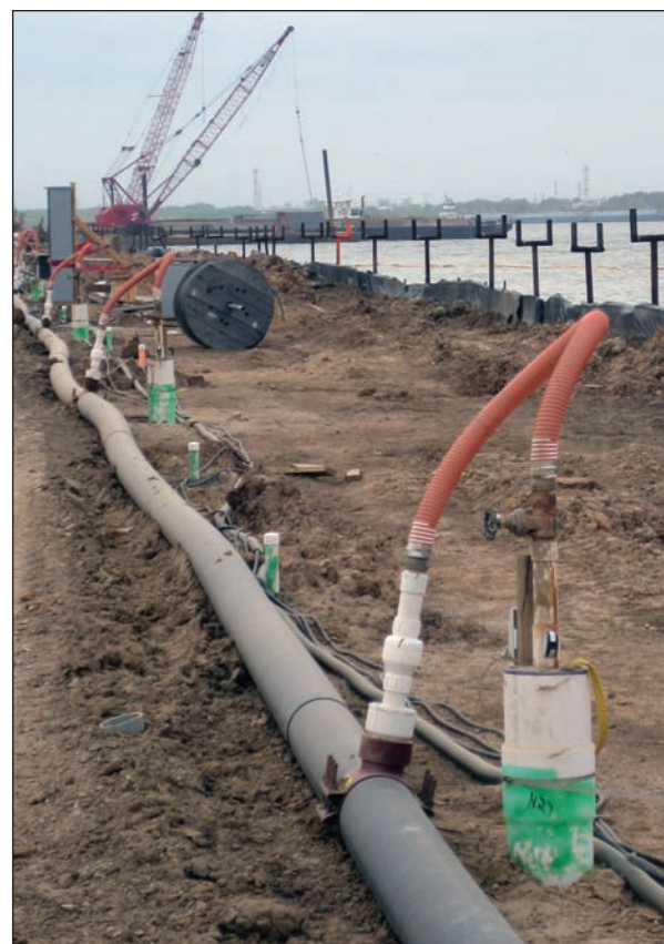
The deep well system at Bayport Container Facility located in the Port of Houston in Texas was a big project that utilized dewatering.
