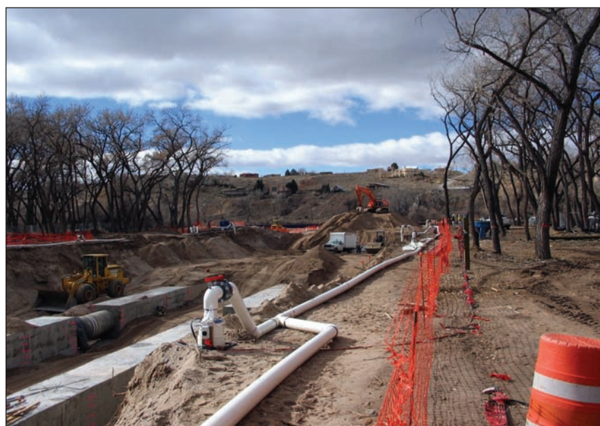
Pipe is installed in the deep well system on the Rio Grande river crossing project in Albuquerque, New Mexico.
