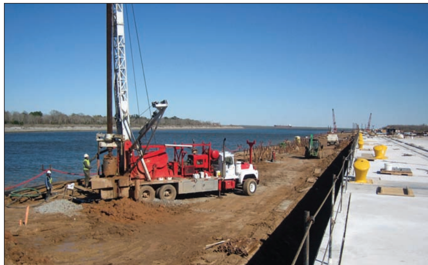
A deep well installation takes place at the Bayport Container Facility in the Port of Houston in Texas.
