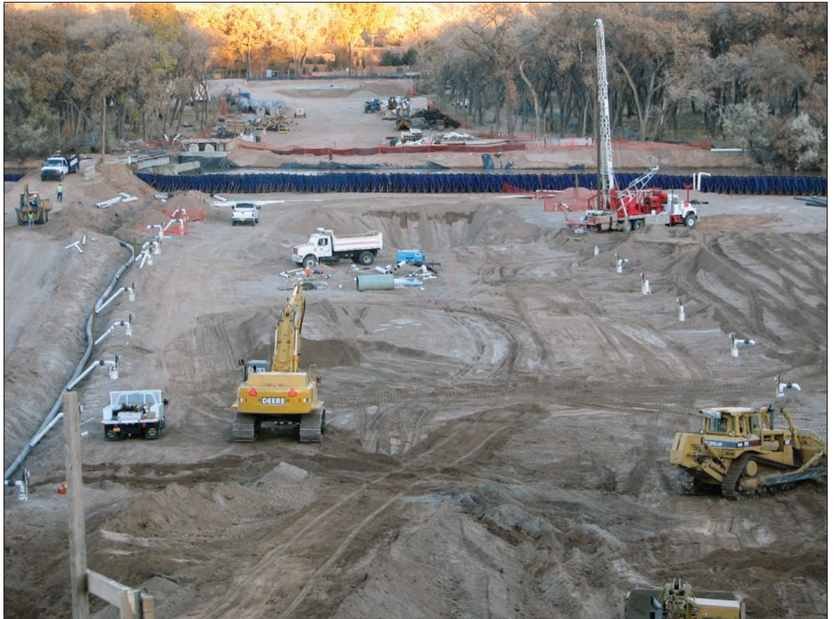
An overview of a deep well system installation in the Rio Grande riverbed in Albuquerque, New Mexico, shows off the great size of the project.
